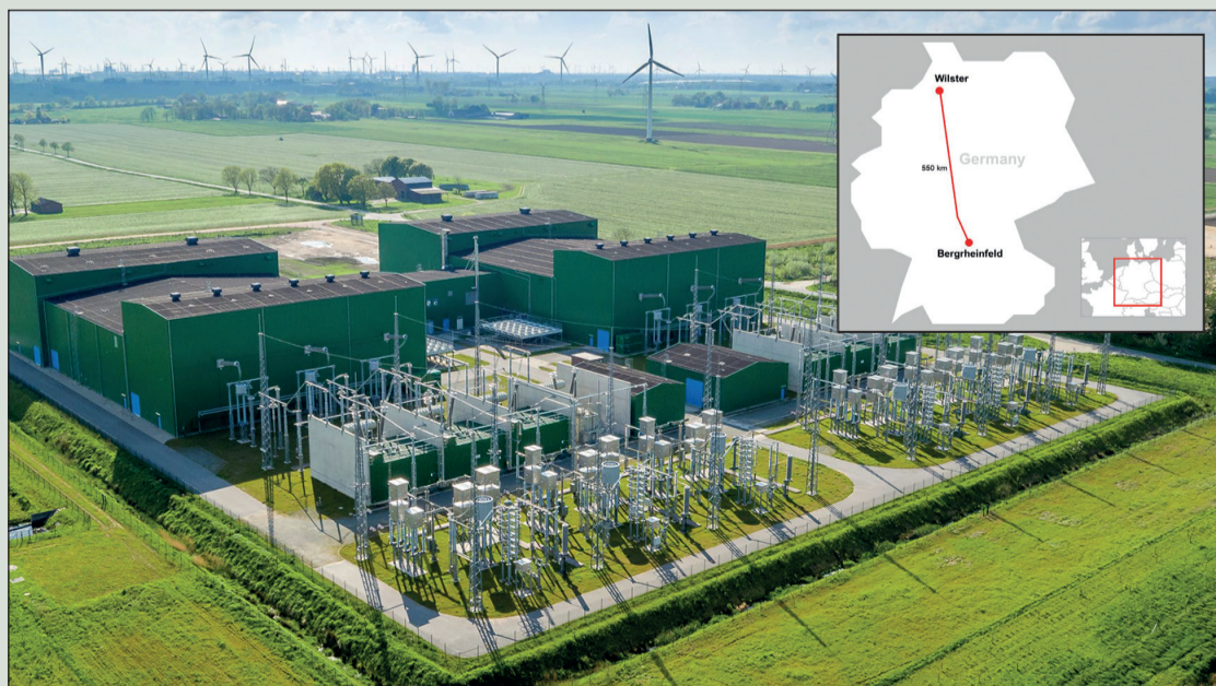
Wilster HVDC converter station. SuedLink DC4 will transmit electricity between Wilster in the north and Bergheimfeld in the south
