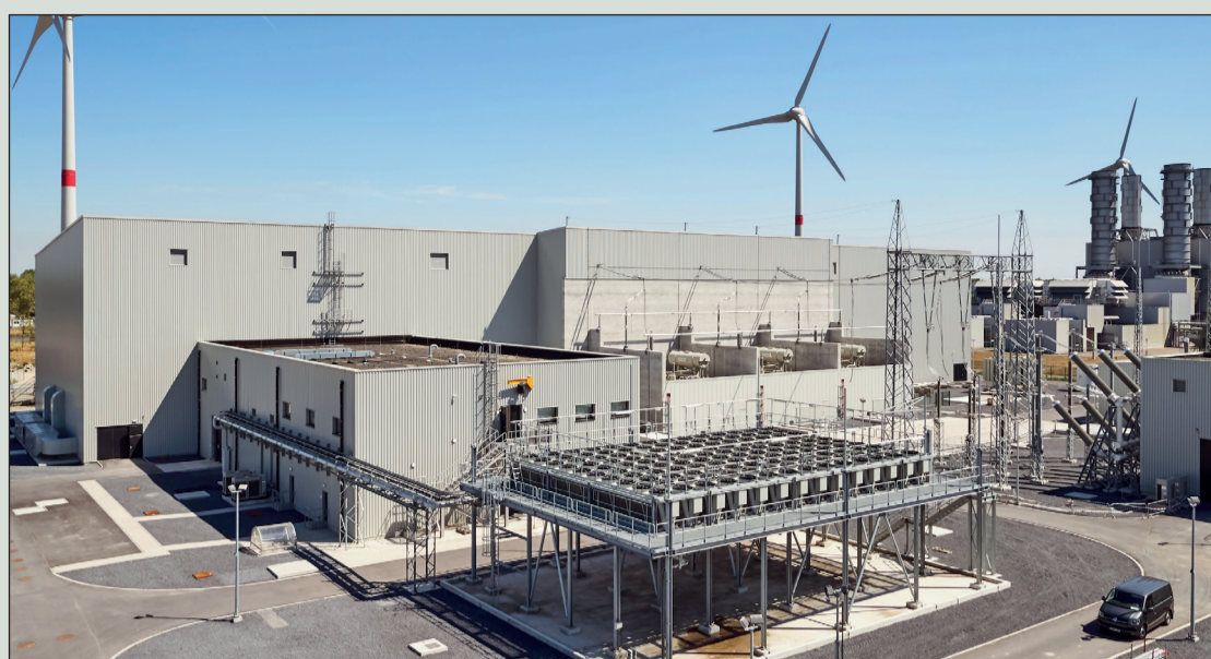
NemoLink converter station: HVDC is crucial to facilitate the integration of wind while maintaining grid reliability and stability
