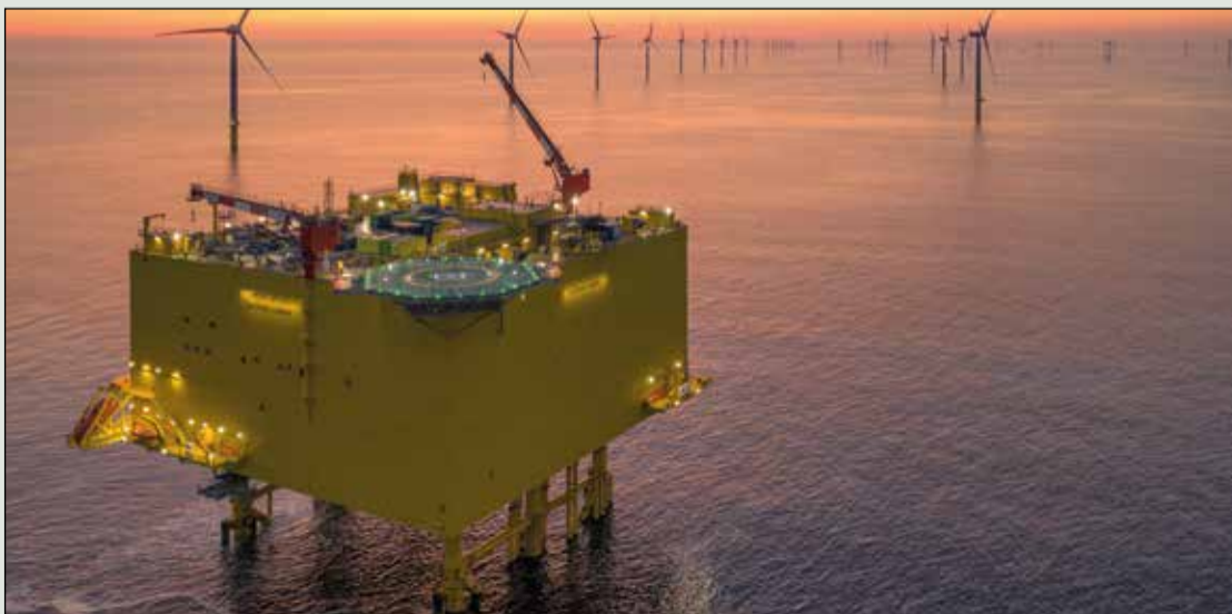
Borwin 3: Siemens Energy is currently building its seventh offshore HVDC connection platform for TenneT in the North Sea
