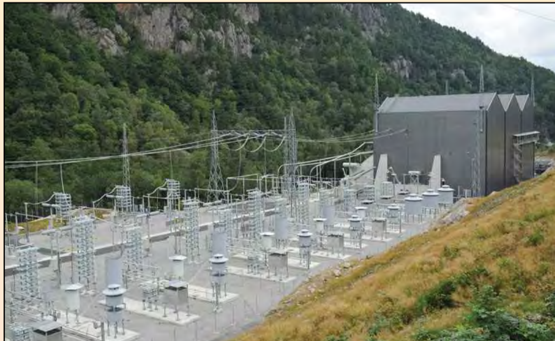
The Feda HVDC converter station is situated in a valley in southern Norway
