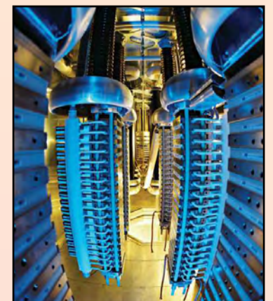
HVDC Light valves: BP will use the technology to power its new Valhall platforms
