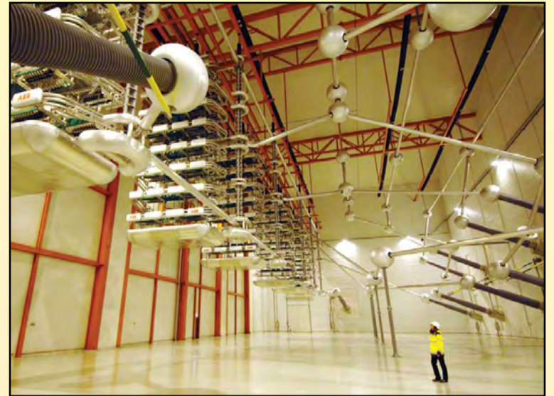
The valve hall at the Feda converter station in Norway is part of the NorNed HVDC transmission link. The valves convert electricity from AC to DC for long-distance, low-loss power transmission. A similar station at the other end of an HVDC link converts DC back into AC electricity
