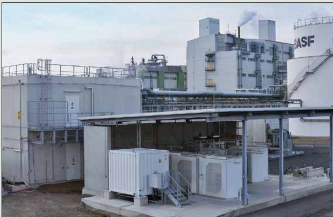
Battery energy storage at the BASF plant will provide black-start capability
