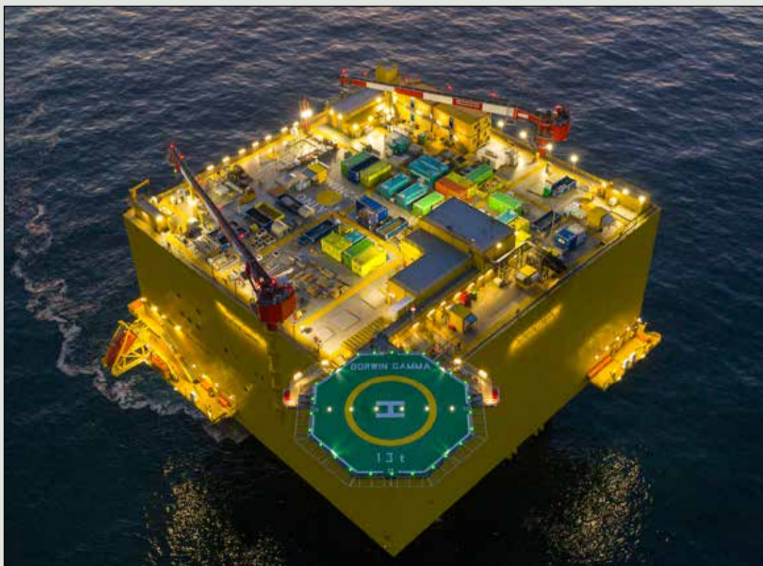
Converter platform of the BorWin3 grid connection in the German North Sea. The grid connection system BorWin3, which can bring 900 MW of wind energy onshore, began operation in August 2019
