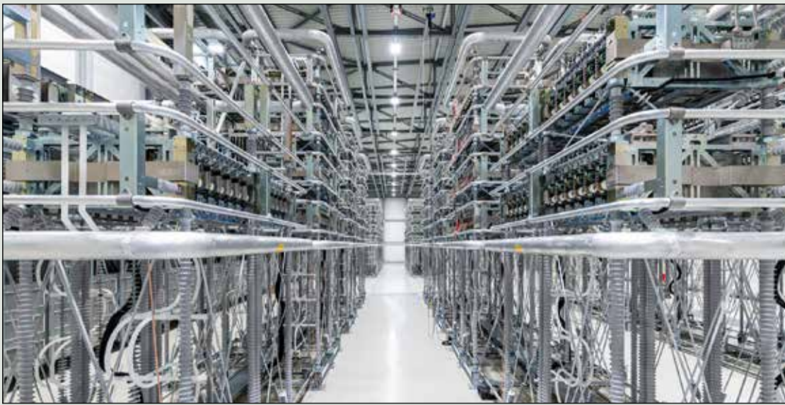
Inside a high-voltage direct current converter hall
