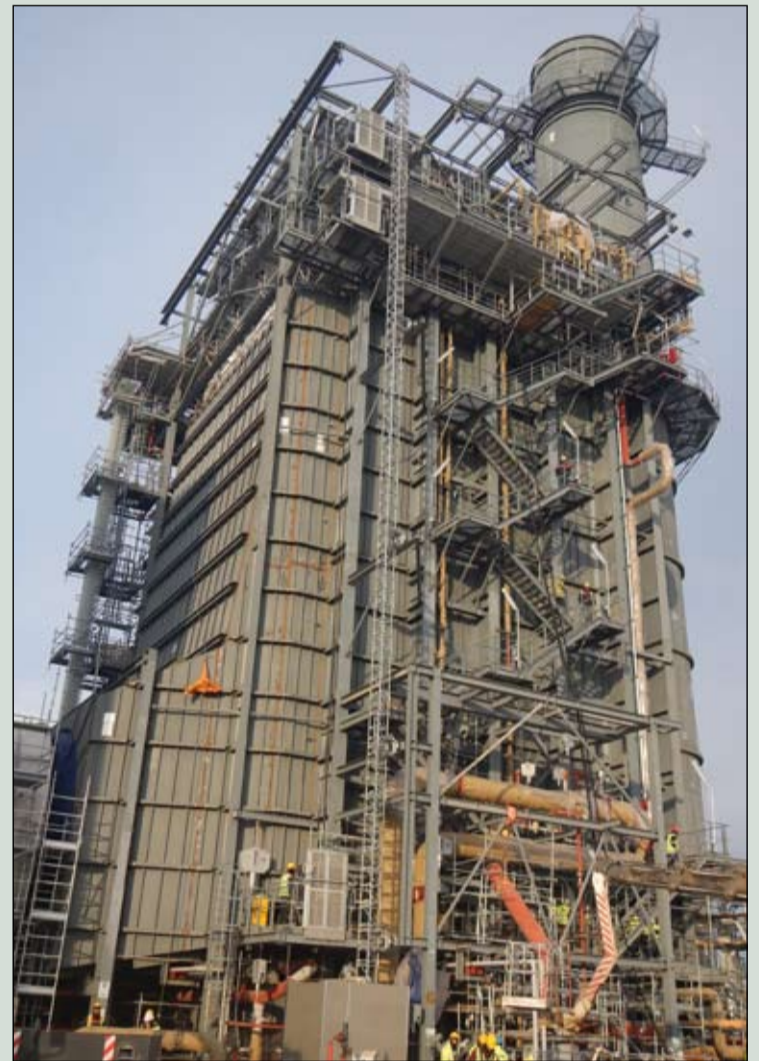
Construction of CMI's HRSG at Hamitabat: the boiler uses stainless steel tubes for an operating steam temperature of 600°C for both high pressure superheater and reheater
