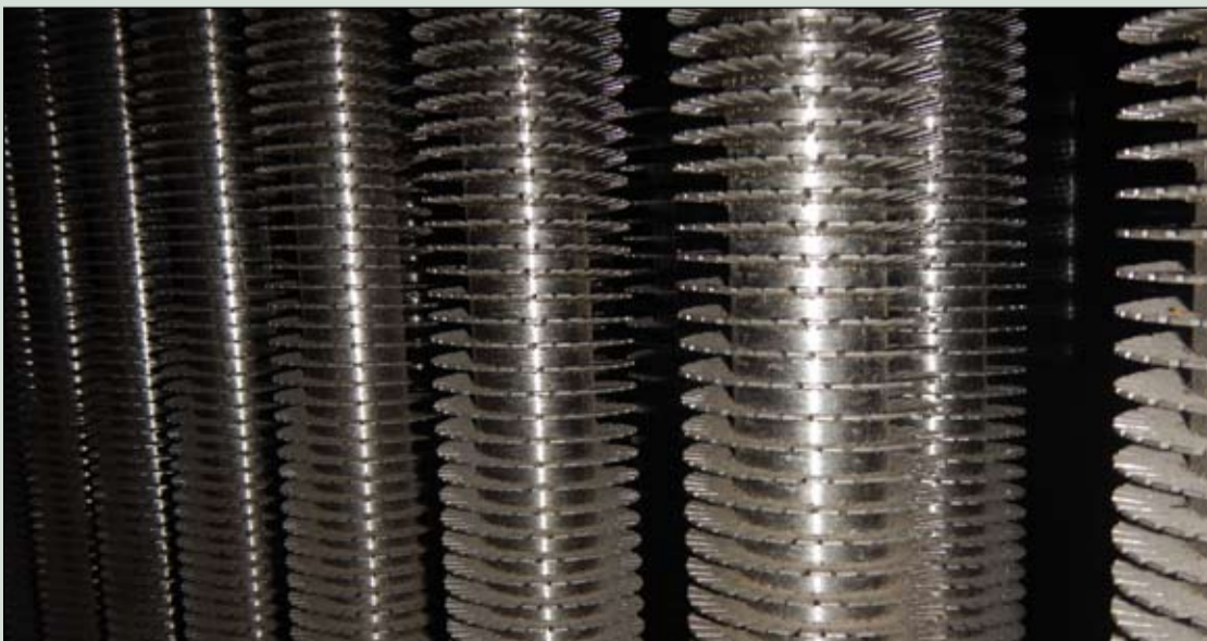
Stainless steel superheater tubes. The shiny surface indicates that it is not carbon steel
