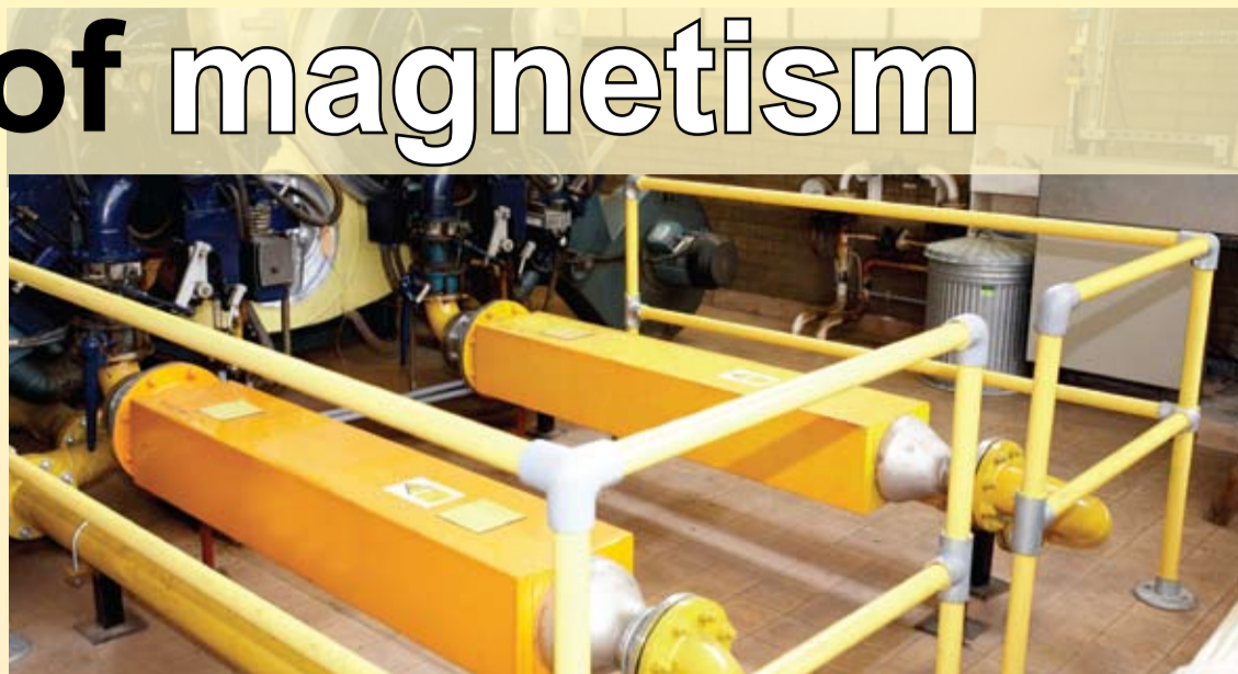
Installation of the system at the sites owned by companies such as Union Papertech has attracted the attention of energy utilities
