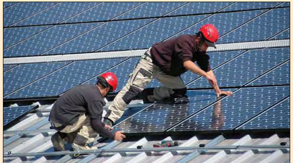
Rooftop installation: high efficiency is particularly important in the residential market
