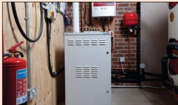
BlueGen installation at Madeley Centre in Staffordshire, UK
