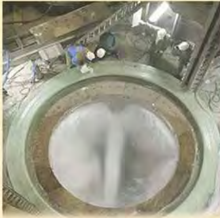
Final tests at the Bushehr plant were completed last month
