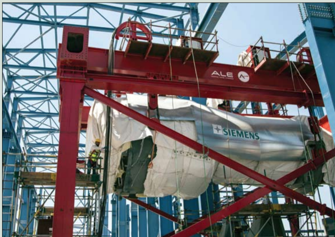
One of four 400 MW gas turbines arriving at the Beni Suef power plant
