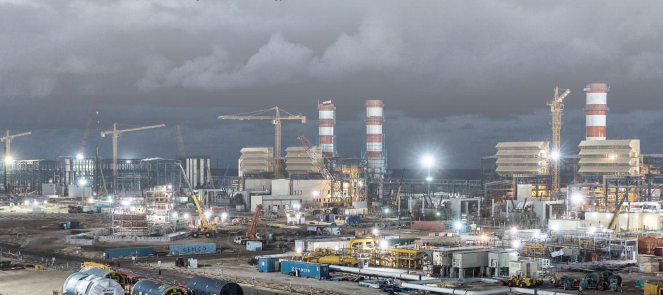
Burullus at night: one of three giant 4.8 GW CCGT plants under construction in Egypt
