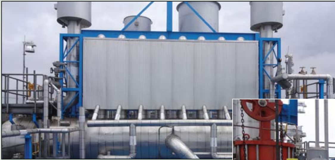
The bottles for secondary water/steam separation are enclosed in one rectangular insulating box
