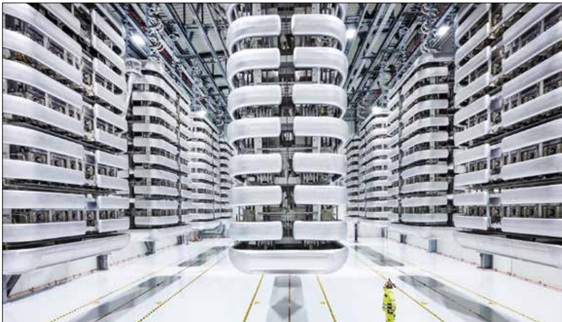
An HVDC valve hall. The integration of renewables often through the use of HVDC links is an important application for power electronics
